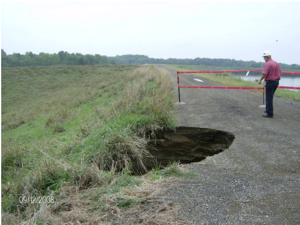
View of Sinkhole Looking Northwest Along Dike
