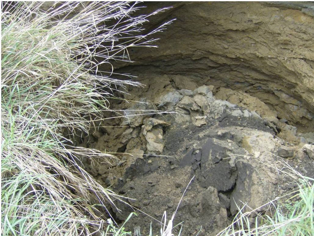
View of Bottom of Sinkhole
